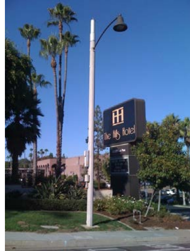
Figure 4: Omni-Directional antenna Courtesy of Crown Castle
