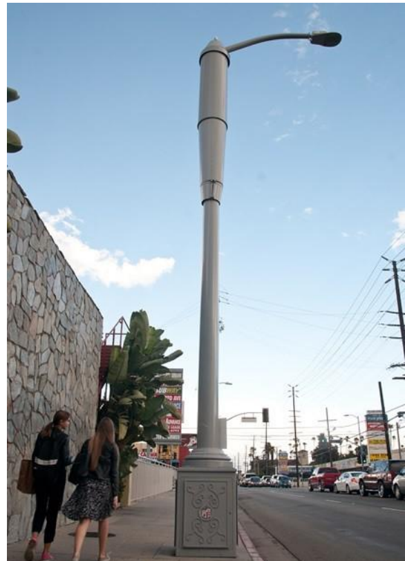
Small Cell integrated into light pole
